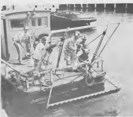
MARINE-FLOATING Equipment Division launch men position the rake used to clear the harbor floor of sea grass and moss. TRAHADORNAN ARUBA lancha di Marine-Floating Equipment Division ta posiconá e halakó cu ta worde usá pa limpia bota di haaf.
